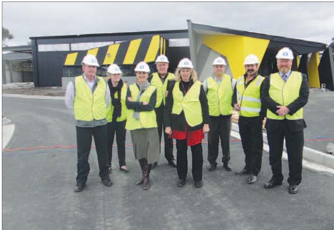
Members of the Bridgewater Trade Training Centre consortium recently inspected progress at the new centre. A community open day to launch the centre is planned for October 20. From left, Wilson Forward (Tas Polytechnic), Jo Harris (Bridgewater and New Norfolk High School pathway planner), Lana Hegol (Tas Polytechnic), Stuart Harvey (Department of Education), Cluny Addis (Bridgewater High School), Simon Nuss (Tas Polytechnic), Shane Hickey (Tas Polytechnic) and Malcolm Elliot (New Norfolk High School).
